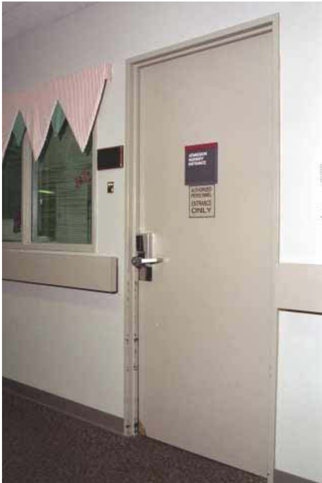
Figure 28-2 Security measures in the postpartum unit and nursery always are in force.
